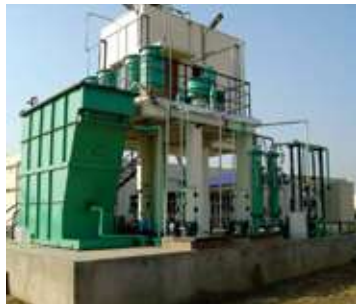
EFFLUENT TREATMENT PLANTS
